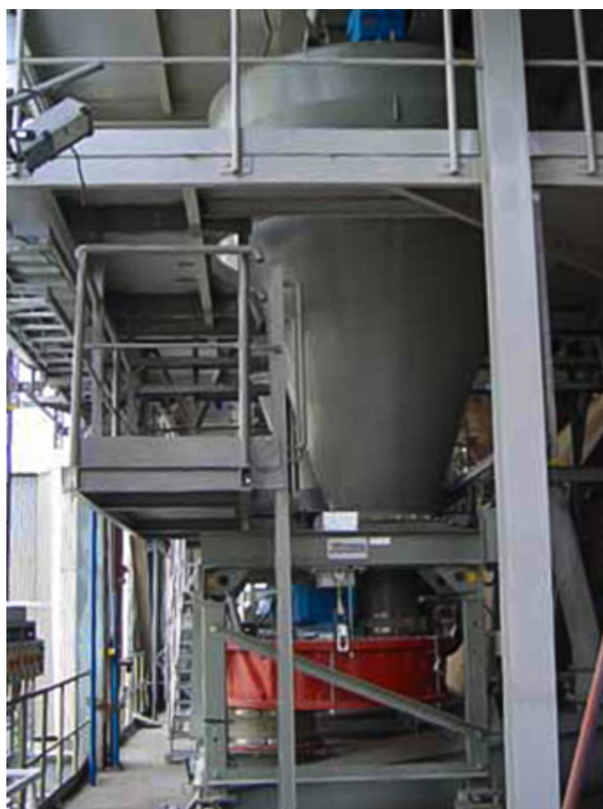
Pfister® TRW-S in the pre-heater tower to the pre-calciner
