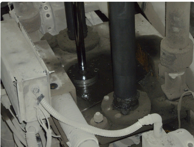
Example of a poorly maintained CARICAMAT®
