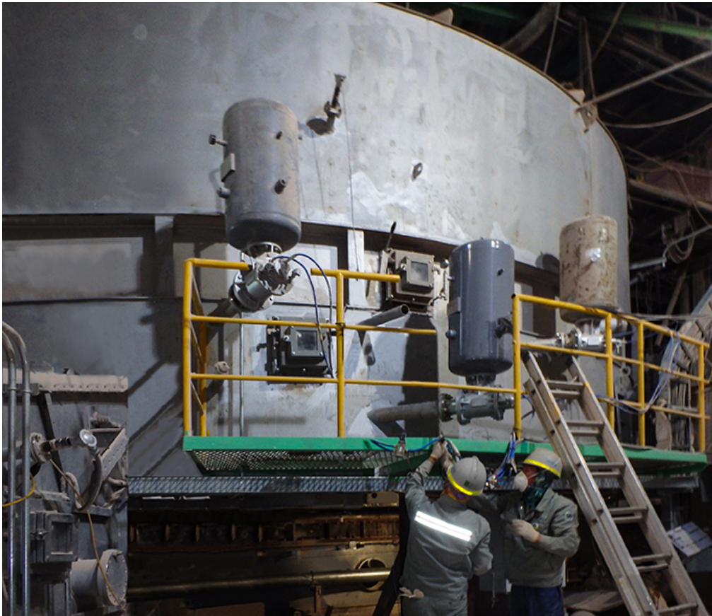
One of the HOTDISC-S reactors installed by Ssangyong
