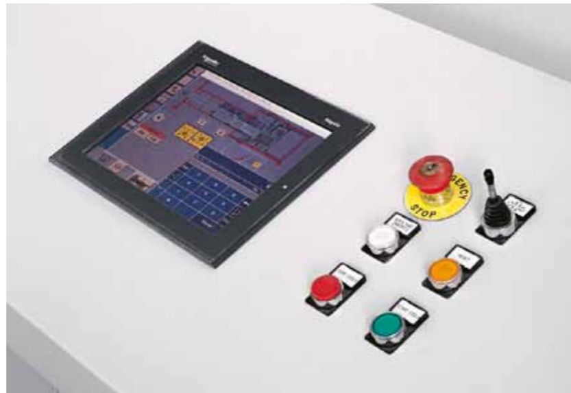
New operator panel
