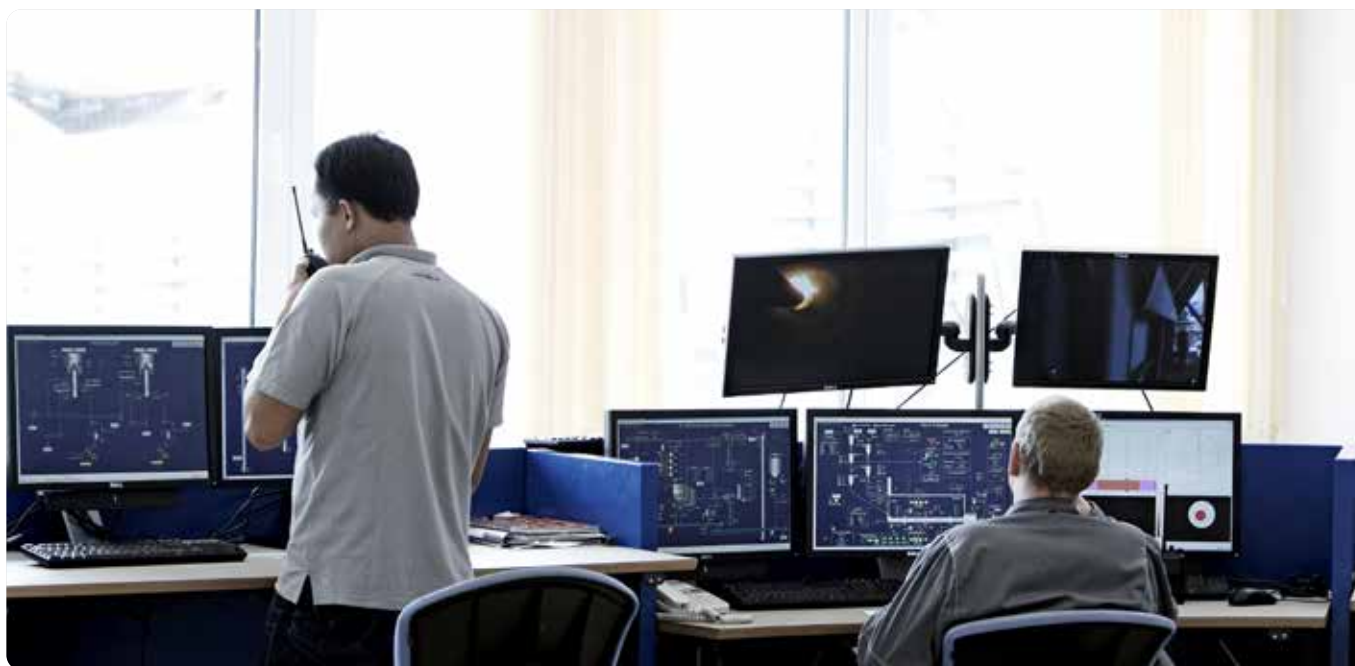
ECS Control Center
